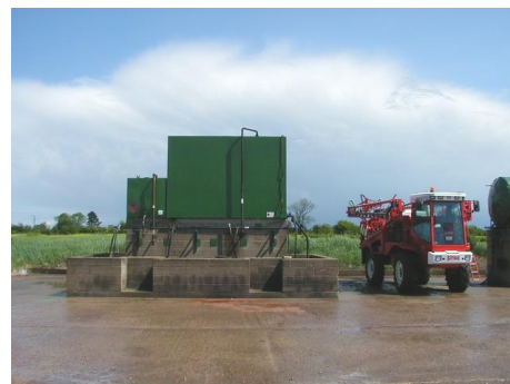
Compliant gravity fed system
