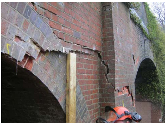
Figure 2 – Damage to farm access bridge in Kent
