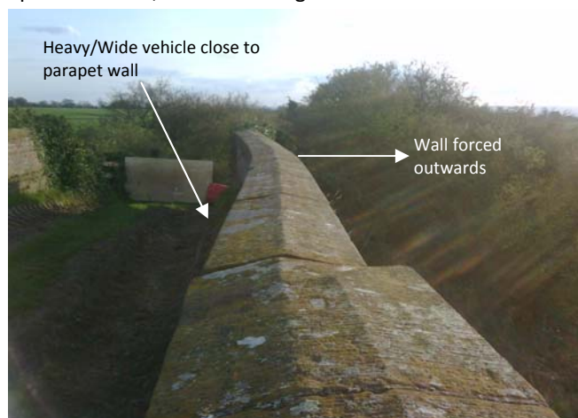
Figure 3 – Typical movement to parapet
