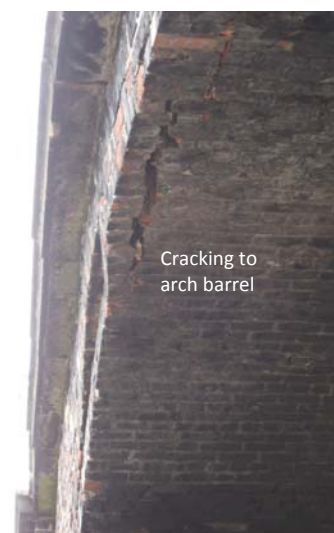
Figure 4 – Cracking around the arch
