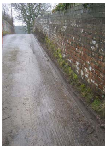
Figure 5 – Cracking and depressions to road surfacing
