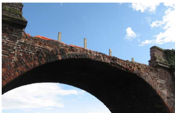
Figure 1 – Damage to farm access bridge at Chester
