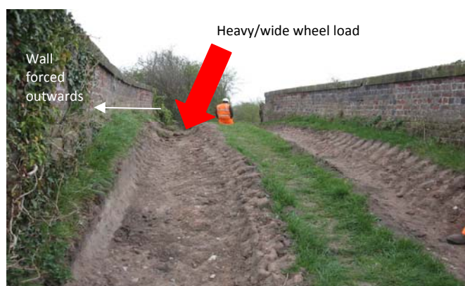
Figure 6 – Typical wheel ruts forcing parapet wall outwards
